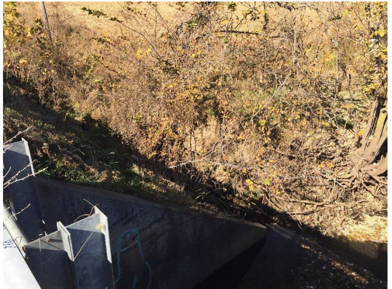
Northeast corner of the structure taken from the roadside. Note the steepness of the grade to the roadside ditch.
