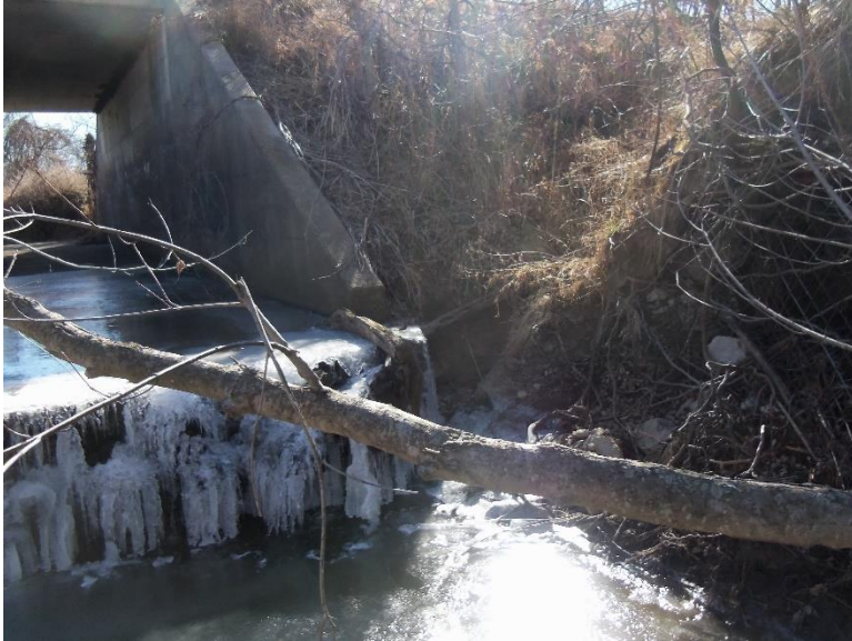
The downstream toewall has degraded to the point that the reinforcing steel is exposed. Note the roadside ditch entering streamway behind the northwest wingwall.
