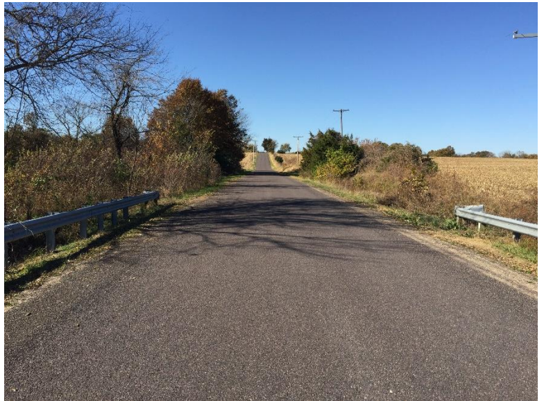
Looking west along Stoenner Road from the structure. The roadway is chip sealed with minimal grass shoulders. Roadside ditches get steeper as they approach the structure. Guardrail has been installed.
