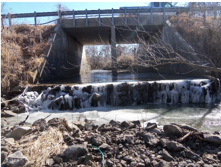
Looking at the downstream end of the structure. There is a significant drop from the end of the apron to the actual stream bottom.
