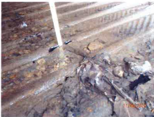
Example of Hole in Bottom of Culvert w/ Undermining
