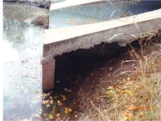
Scour Void behind Concrete Headwall
