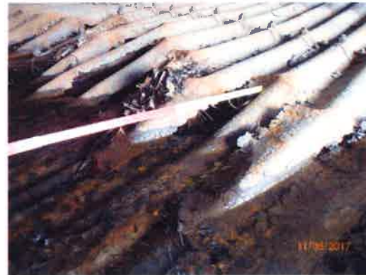
Typical Deterioration in Bottom of Pipe
