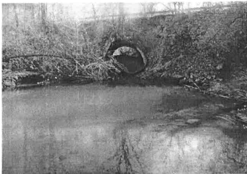
Picture of collapsed culvert outlet and scour pool
