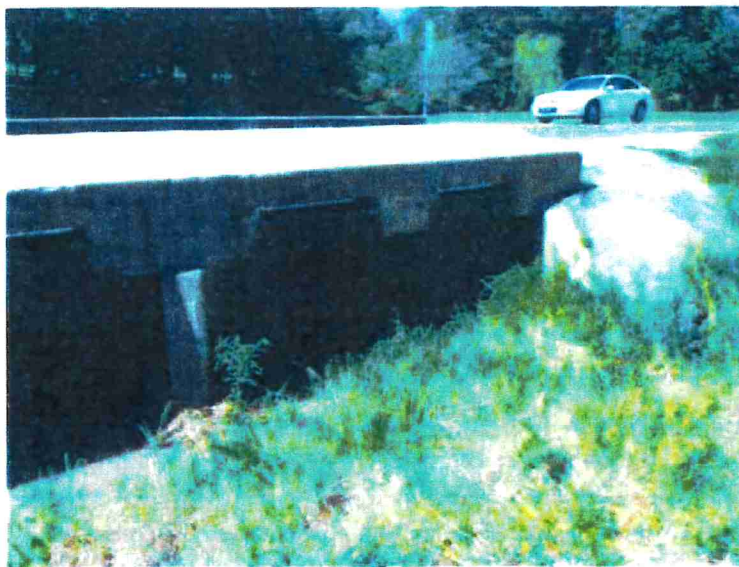
July 2017 site photo of the southeast corner of the structure. Note the paving adjacent to the RCB to prevent erosion created by runoff from the roadway surface.
