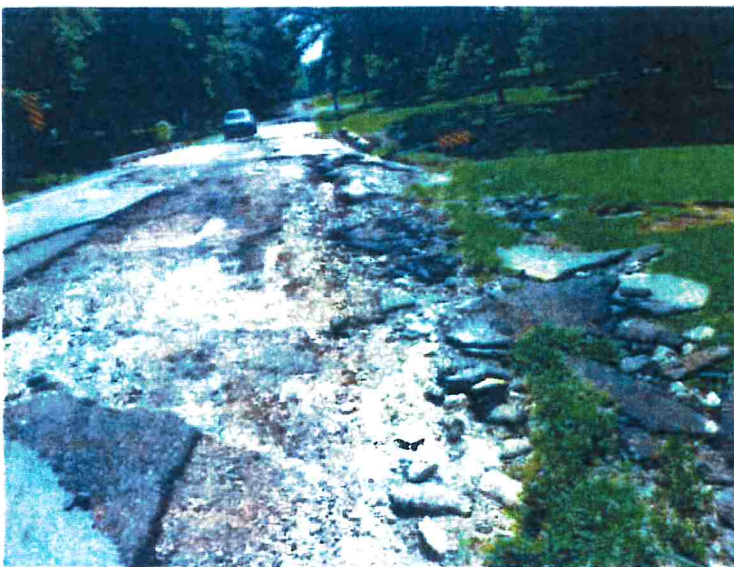
July 2019 flood damage to roadway (looking at road and ditch west of the structure).
