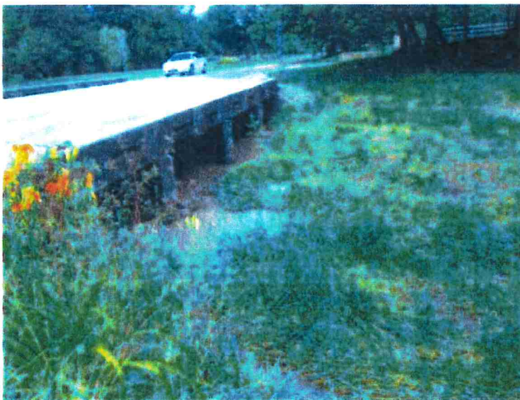
July 2017 site photo of the upstream side of the structure. Note the west bank is partially blocking the far cell from carrying full capacity flows.
