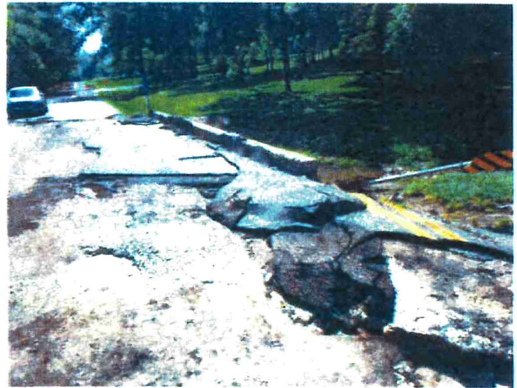
July 2019 flood damage to bridge and roadway (looking at southwest corner of structure).
