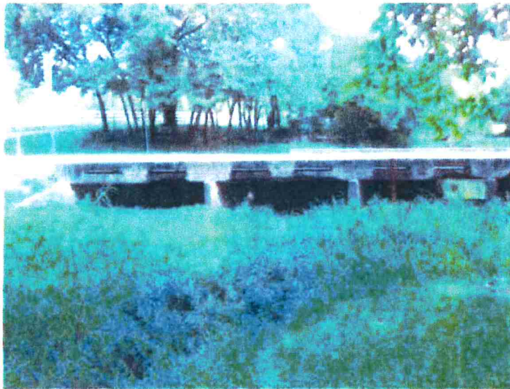
July 2017 site photo of the downstream side of the structure. Note bank on the left side of photo possibly impeding the flow through the outside cell.
