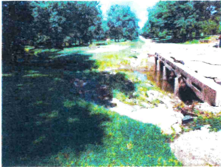
July 2019 flood damage (looking west towards downstream side of structure).
