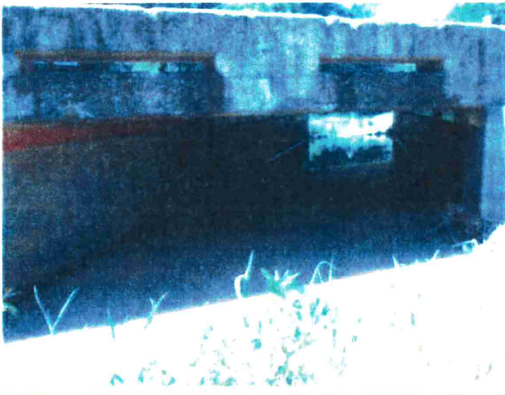
July 2017 site photo of the typical curb/railing along the bridge. The concrete is in very poor condition.
