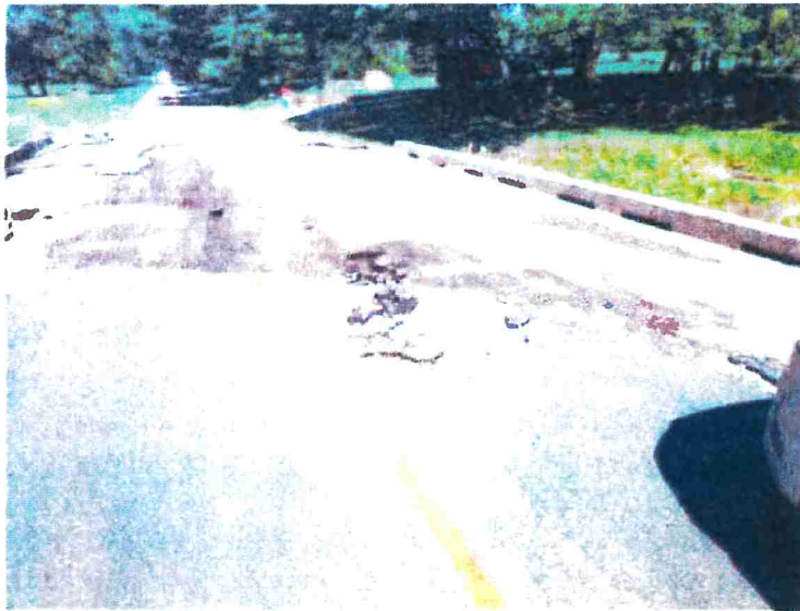
July 2019 flood damage to bridge deck (looking west from the east side of structure).
