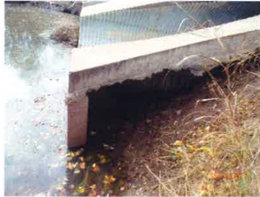
Scour Void behind Concrete Headwall
