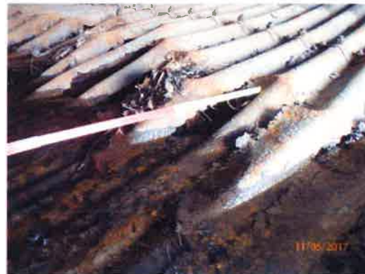
Typical Deterioration in Bottom of Pipe
