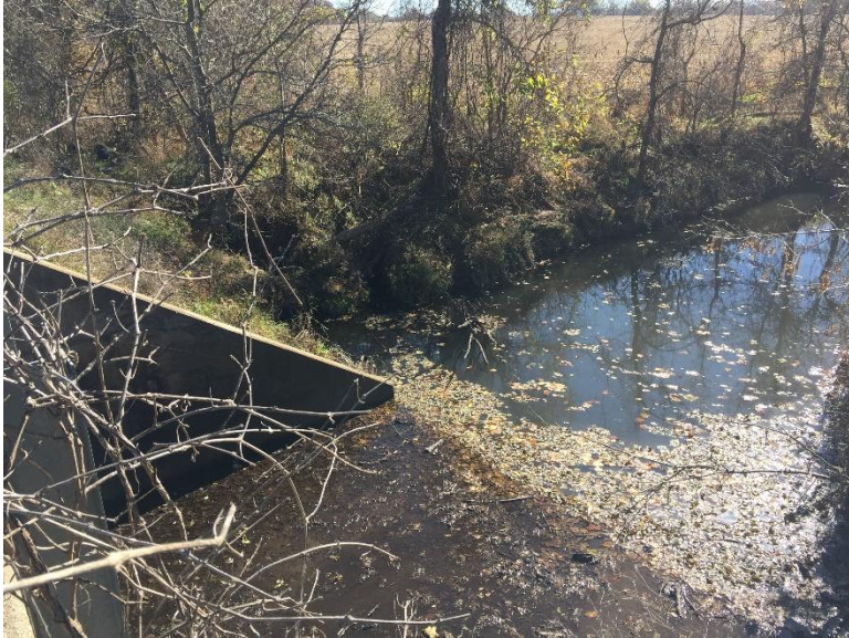
Upstream end of the structure. No center wingwall was constructed. Note the erosion of the roadside ditch at the end of the southeast wingwall. Rock blanket should be considered for each of the locations where the roadside ditches enter the streamway to prevent erosion.
