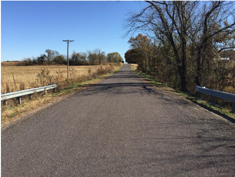
Looking east along Stoenner Road from the structure The roadway is chip sealed with minimal grass shoulders. Roadside ditches get steeper as they approach the structure. Guardrail has been installed.
