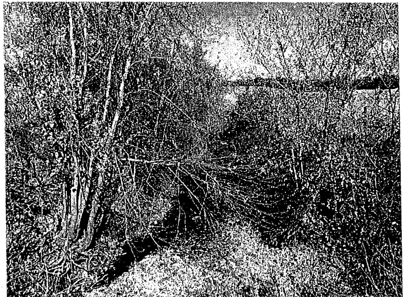
Looking downstream from the double cell RCB. The stream banks are very well defined and extend outside the wingwalls of the structure. Note the erosion around the base of the trees immediately downstream of the structure. These should be removed to prevent blockage of the stream if they were to fall during a major storm event.
