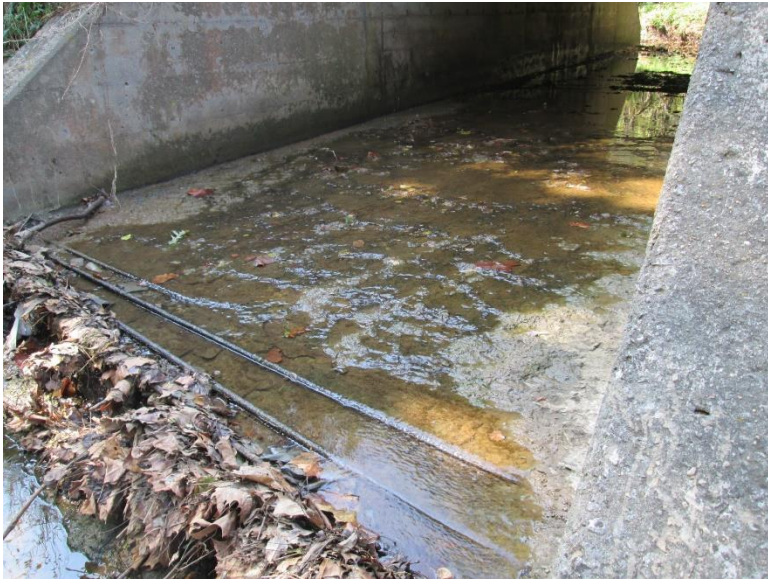
The floor of the culvert is severely damaged. There is exposed reinforcing steel in both cells of the structure.
