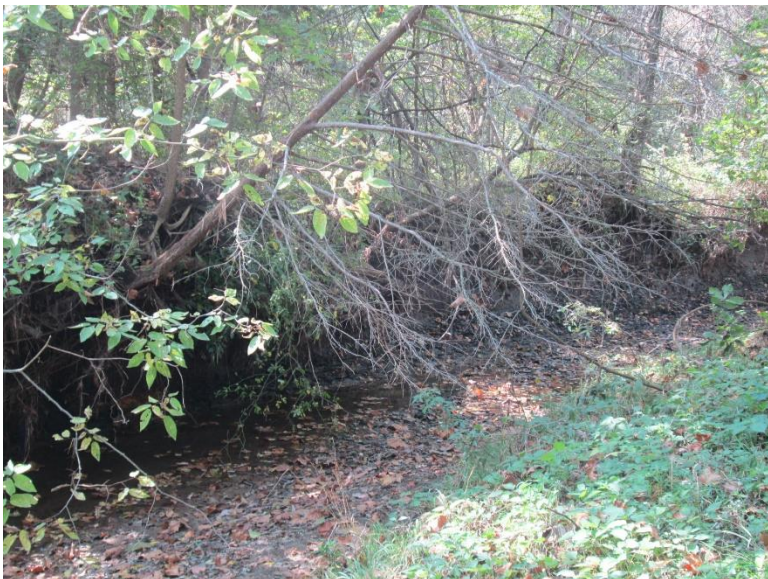
Looking upstream from the structure. The channel is tucked into the bank is directed towards the southerly cell of the RCB. Note the amount of vegetation upstream that will need to be reviewed as part of the environmental clearance.
