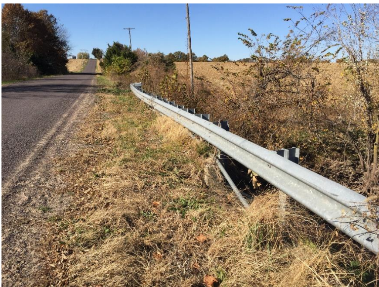
Looking west along the north side of Stoenner Road at the structure. Note the underground utility that crosses over the double cell RCB (assumed fiber optic). During the field visit we noted overhead power and telephone on the poles. We did not see any markers for gas or water at this time. Need to review the County records for private easements.
