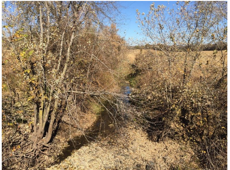
Looking downstream from the double cell RCB. The stream banks are very well defined and extend outside the wingwalls of the structure. Note the erosion around the base of the trees immediately downstream of the structure. These should be removed to prevent blockage of the stream if they were to fall during a major storm event.
